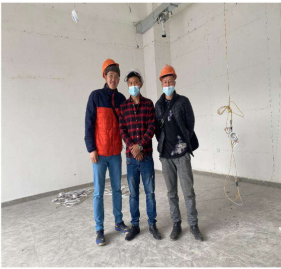
Tengis, on the left, overseeing the repairs of the building where we are planting a new church.
